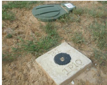
collection chamber and inspection chamber
