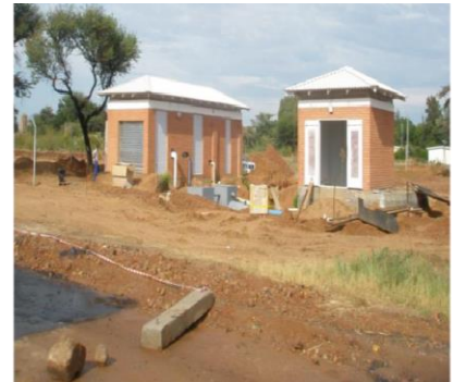
vacuum station with biofilter and genset
