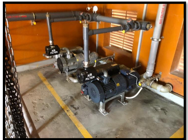
two vacuum pumps
