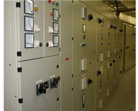
Electrical panels, constructed as per local standards
