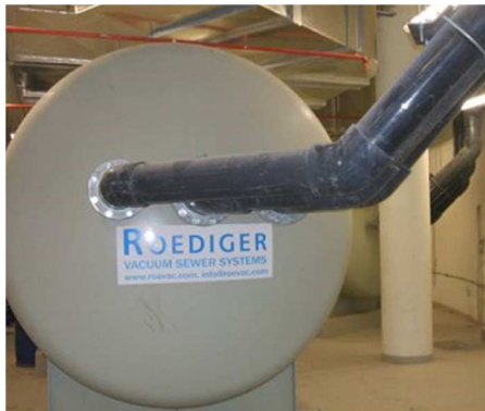
4 vacuum vessels, each of capacity 25 cbm
