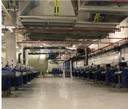
Centralised vacuum station
