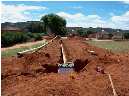
Roediger Collection Chamber under construction with the gravity inlet from a group of houses
