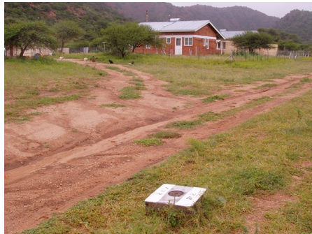
Inspection pipe cover instead of manholes for the vacuum collection pipe underground
